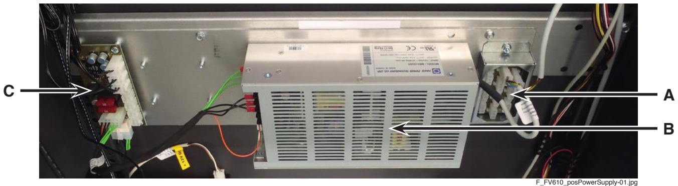
Illustr. 5-3 Position of the power distribution box
